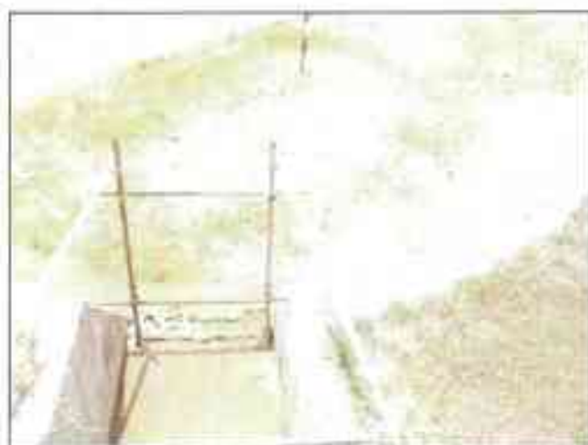
There is no water at SW-5
